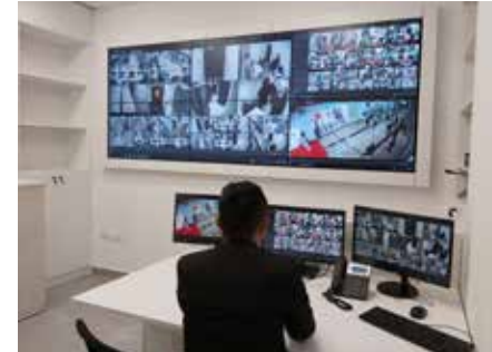
Western Region Security Control Centre, Mumbai, India
